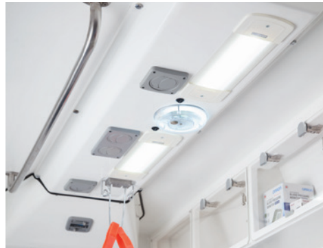
Cabin ceiling services panel
